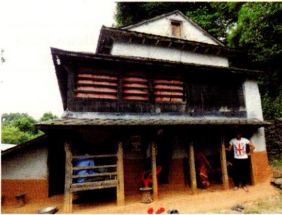
Figure 5.6 A House Categorized as 'Damaged beyond Repair', Which Has No Serious Damage on the Surface
