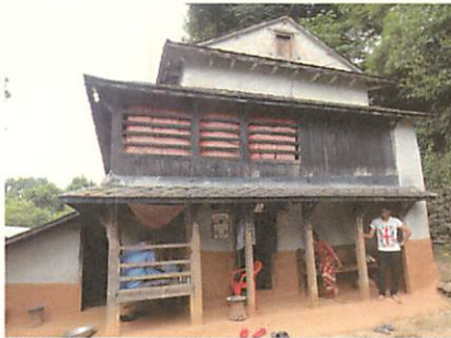
Figure 5.6 A House Categorized as 'Damaged beyond Repair', Which Has No Serious Damage on the Surface
